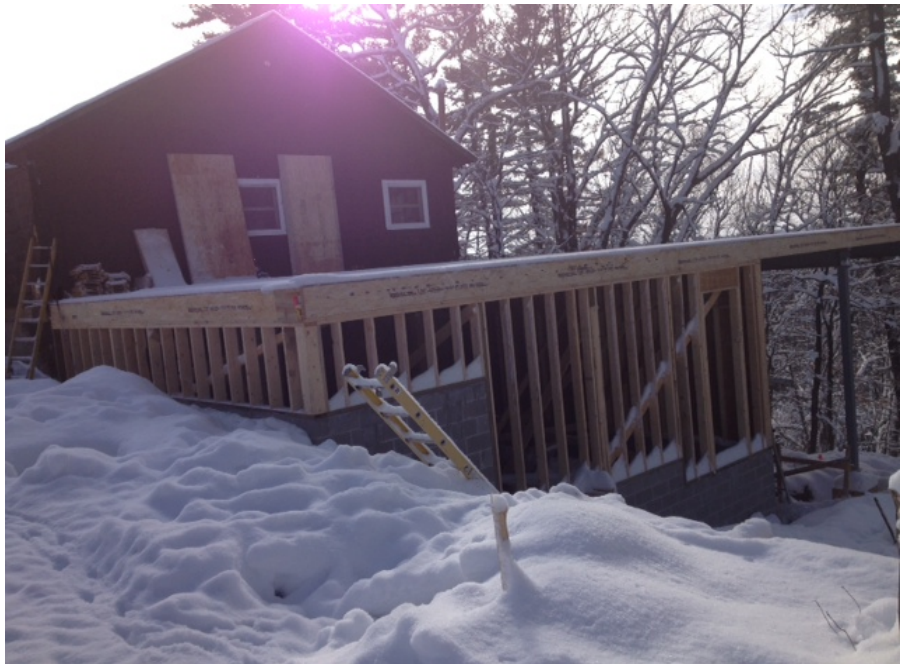
Above you can see that work on the dining hall remodel is progressing nicely. The windows were all boarded over at the time of winter camp, so we couldn't see inside, but I'm sure it will be great – and hopefully cooler in the summer...
